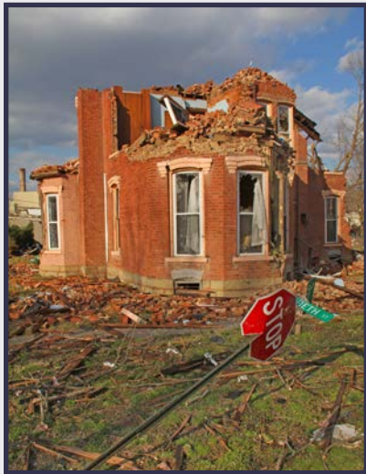
A tornado in Ohio damaged this building.
